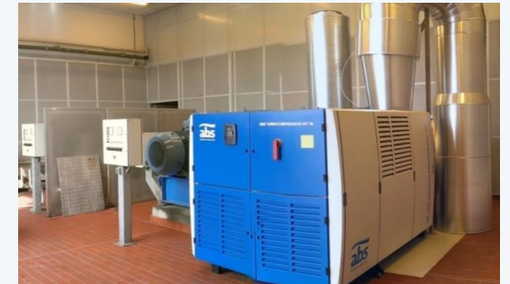
Control of blower
