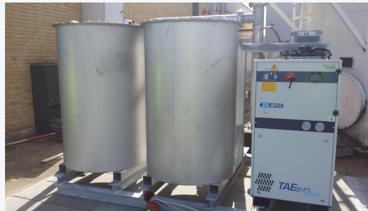
Gas treatment, activated carbon
