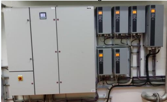
VLT Control of return sludge
