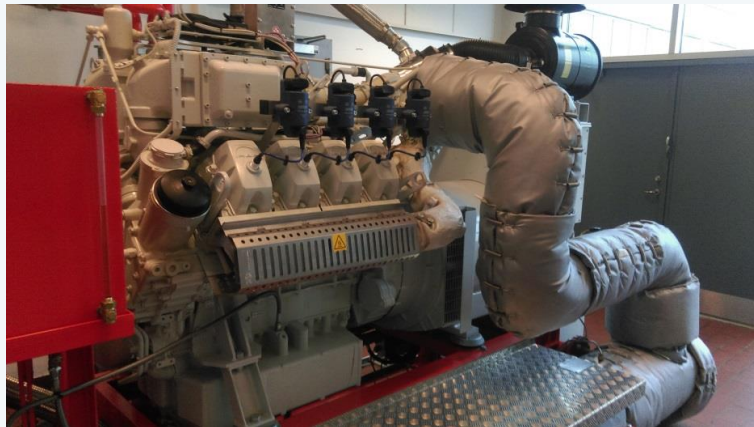
Gas engine installation
