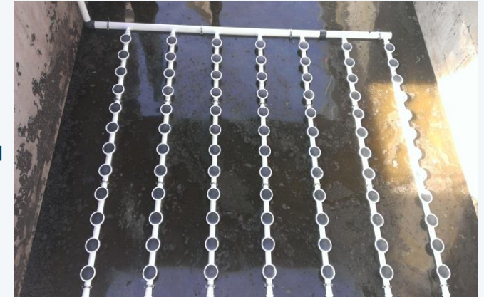
New membranes - fine bubble aeration
